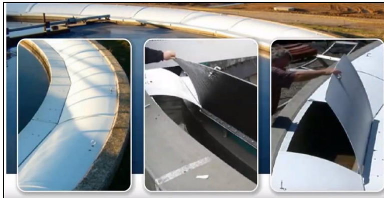
Figure 12 – Clarifier Launder Cover
