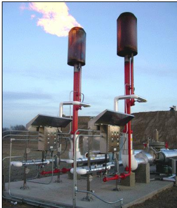
Figure 28 – Waste Gas Flare Example
