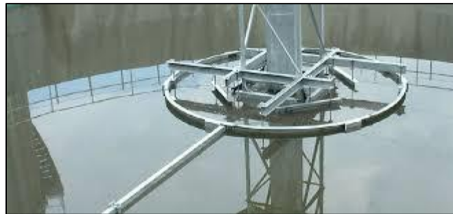
Figure 7 – FEDWA Clarifier Inlet
