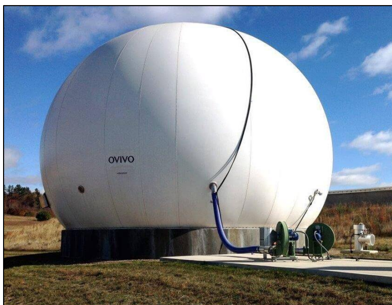
Figure 29 – Remote Biogas Storage Example
