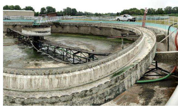
Figure 3 - Final Clarifier Mechanism
