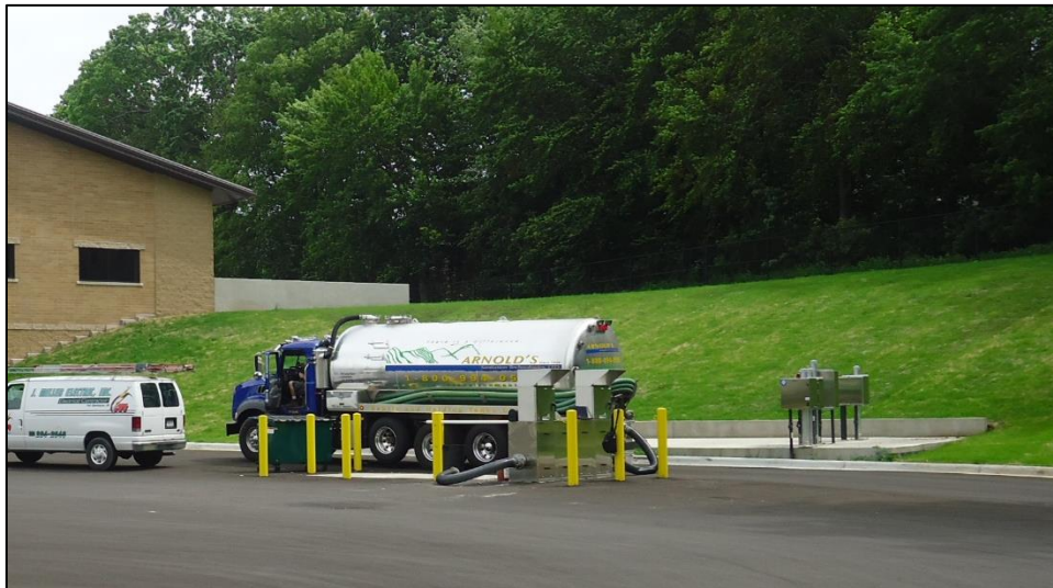
Figure 2 – Septage Receiving Station
