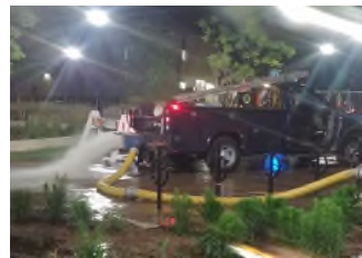
Hydrant Flushing Insuring the integrity of the water system and providing high quality water
