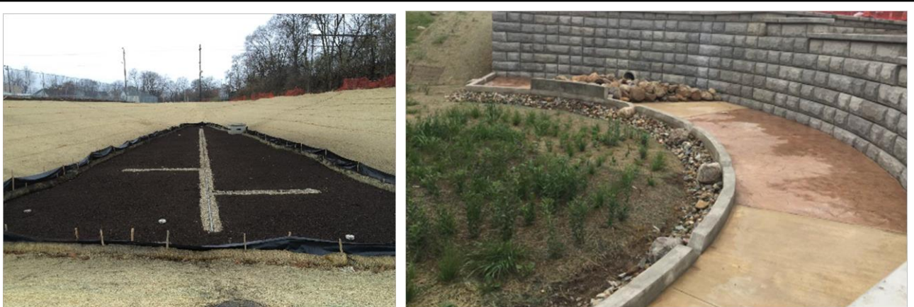
Figure 4.03-2 Enhanced Bioretention Basins in Cleveland, Ohio Serving 19- and 59-Acre Drainage Areas, Respectively
